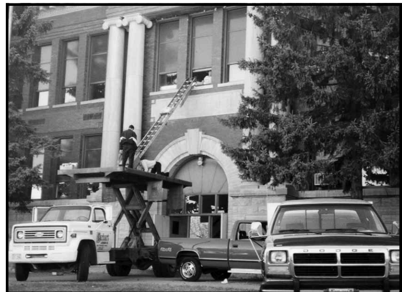
Crews work to removed books, equipment and other articles from the second story of the Middle School prior to the renovation of the building in 2000. The original building once housed all the students attending Wayne Public School.
